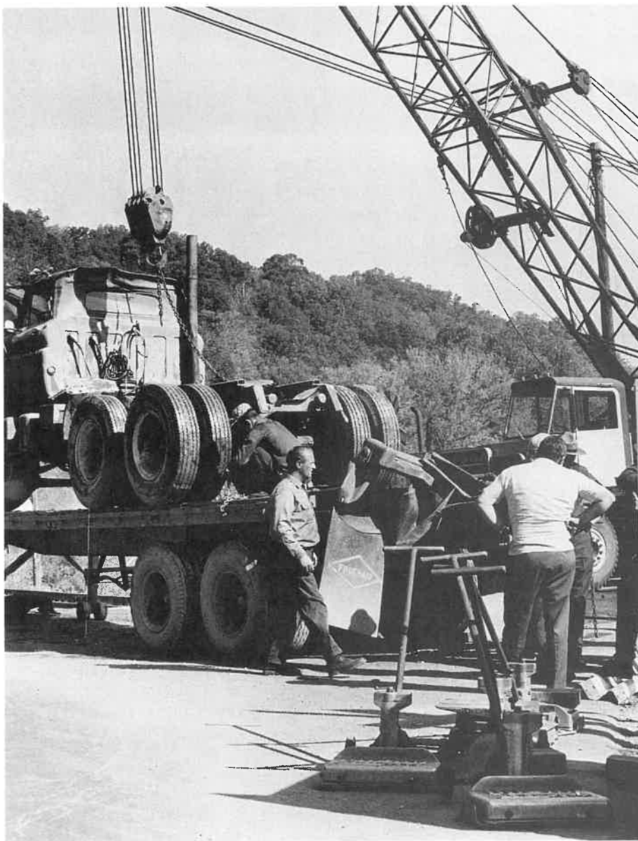
The famous bridge was finally laid low by an overweight truck. Here workers prepare the truck cab for removal from the site. Photographer unknown, courtesy Herald-Dispatch .
